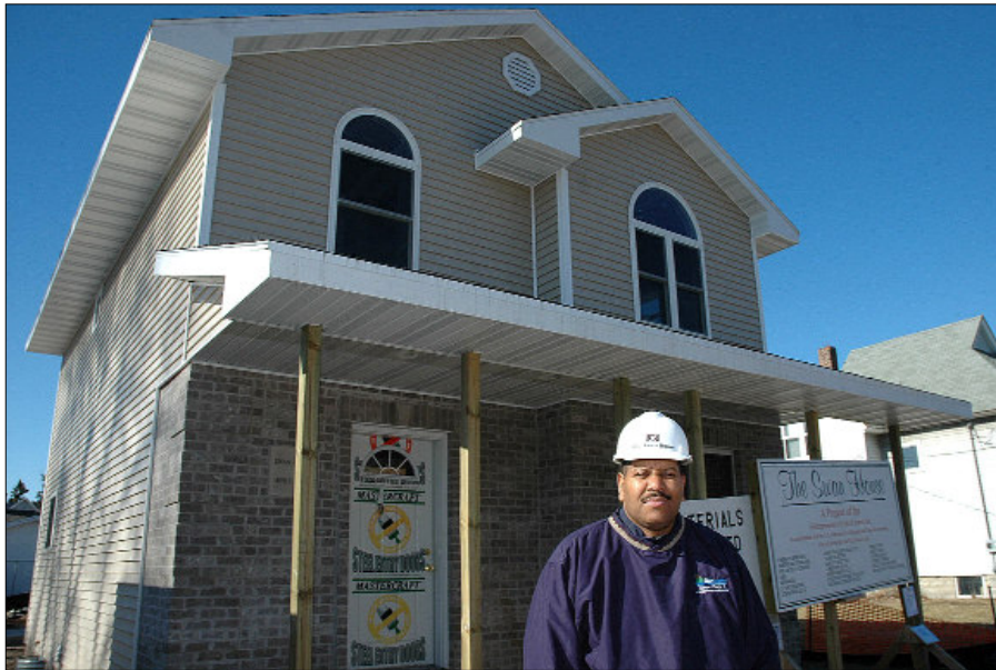
Chris Swan, pictured at the under-construction Swan House at 941 Shawano Ave., is making his difference by coordinating the building of new homes for people who need help with their housing, such as a single parent with children who is pursuing a four-year college degree. The Business News photo by J.A. Robb
